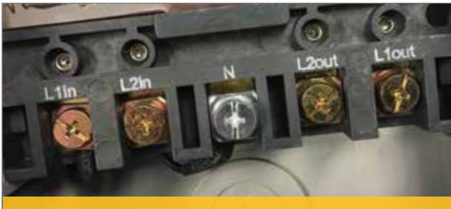
CLEARLY MARKED WIRING TERMINALS
